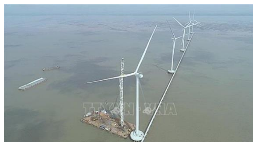
Installing pole propellers at Dong Hai 1 wind power project (Dong Hai district, Bac Lieu province). Illustration: Chanh Da/TTXVN
