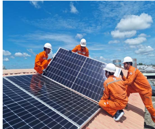
Nearly 99% of rooftop solar power systems in Ho Chi Minh City are installed for on-site self-use. Photo: congnhiepmtruong.vn
